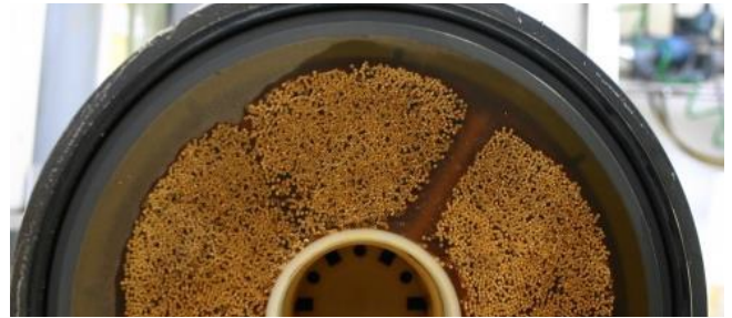
Typical Iron fouling
